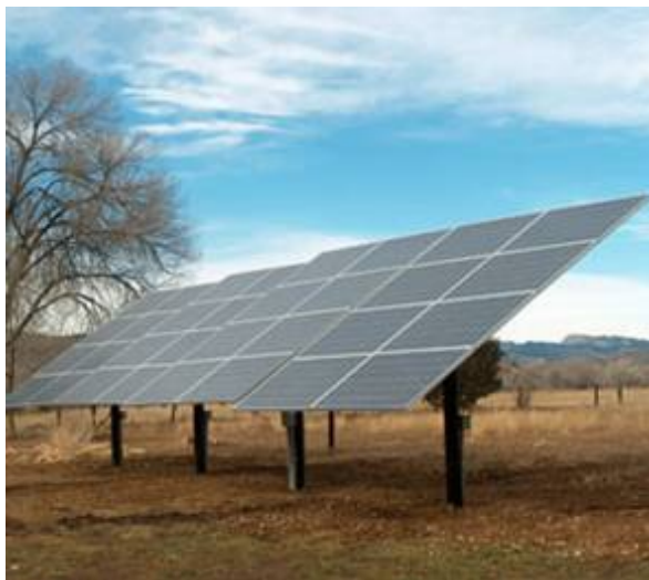
Utility scale power plants
